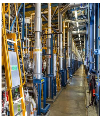
Figure A3: Electrolyzers for chlor-alkali production in Rotterdam
