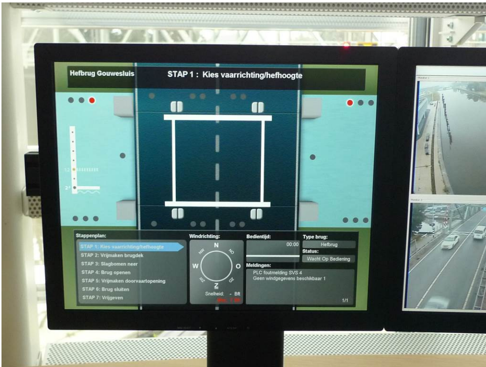
Figuur 11: operator status console
